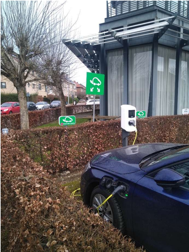
Figure 1 : Charging stations in front of Kraainem 33’s building
